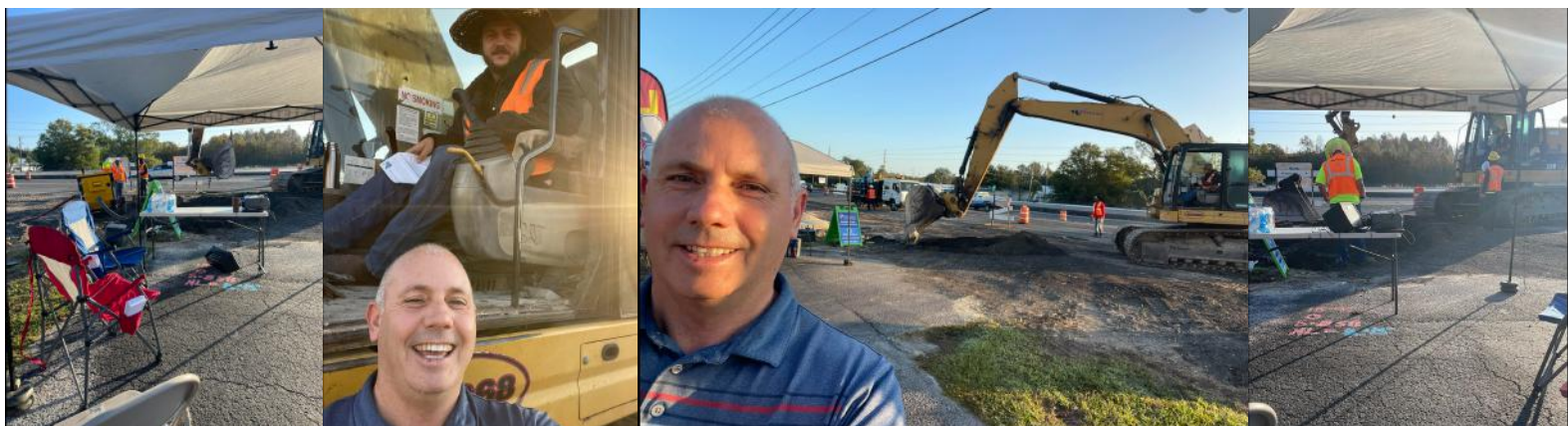
7am Mission outreach in Crystal River The Miracle Center and a excavator is closing the road. This is Austin got to share Jesus with the operator! Prayed with Phil who just lost his 2 year old to drowning! God is moving as I find myself on a road construction site.!
